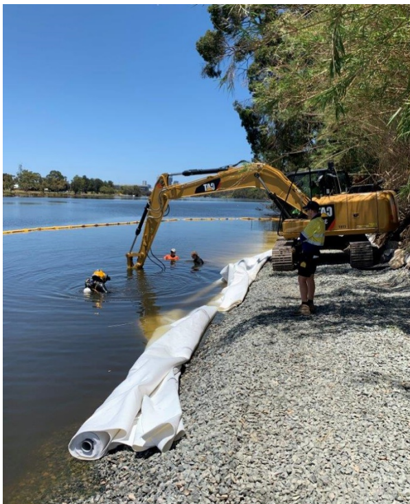
Image: Contractor placing geotextile for the revetment with the assistance of divers.
